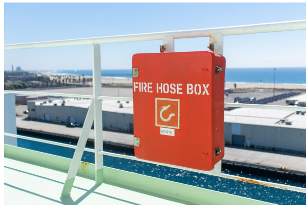
Fire Hose Box on a Vessel at the Port of Hueneme.
